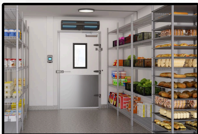
Walk-In Refrigeration Box
