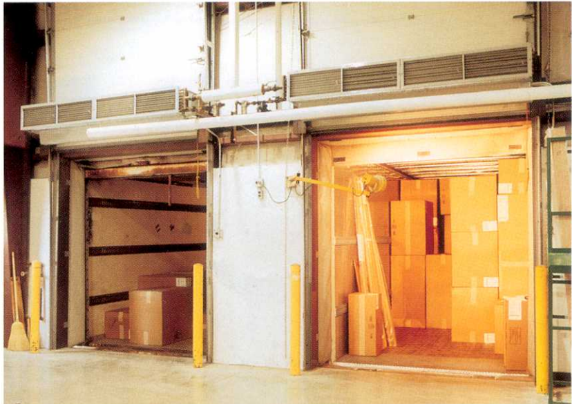
A MOVING BARRIER of air helped keep workers warm and ensured quality control in this warehouse operation.
